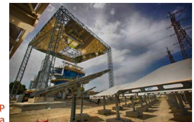
the 2MWth peak load CSP plant at San Filippo del Mela
